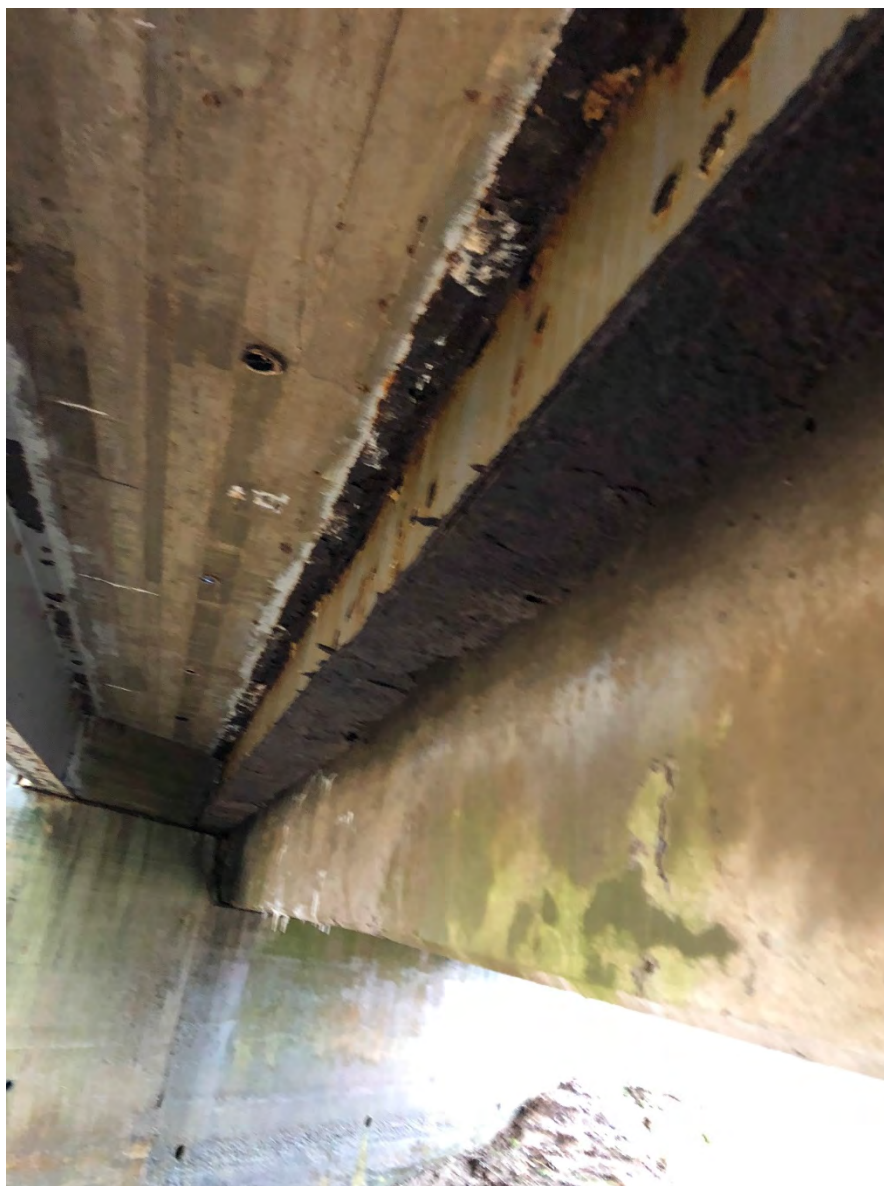
Extensive Corrosion of inner I-Beam at Inlet
