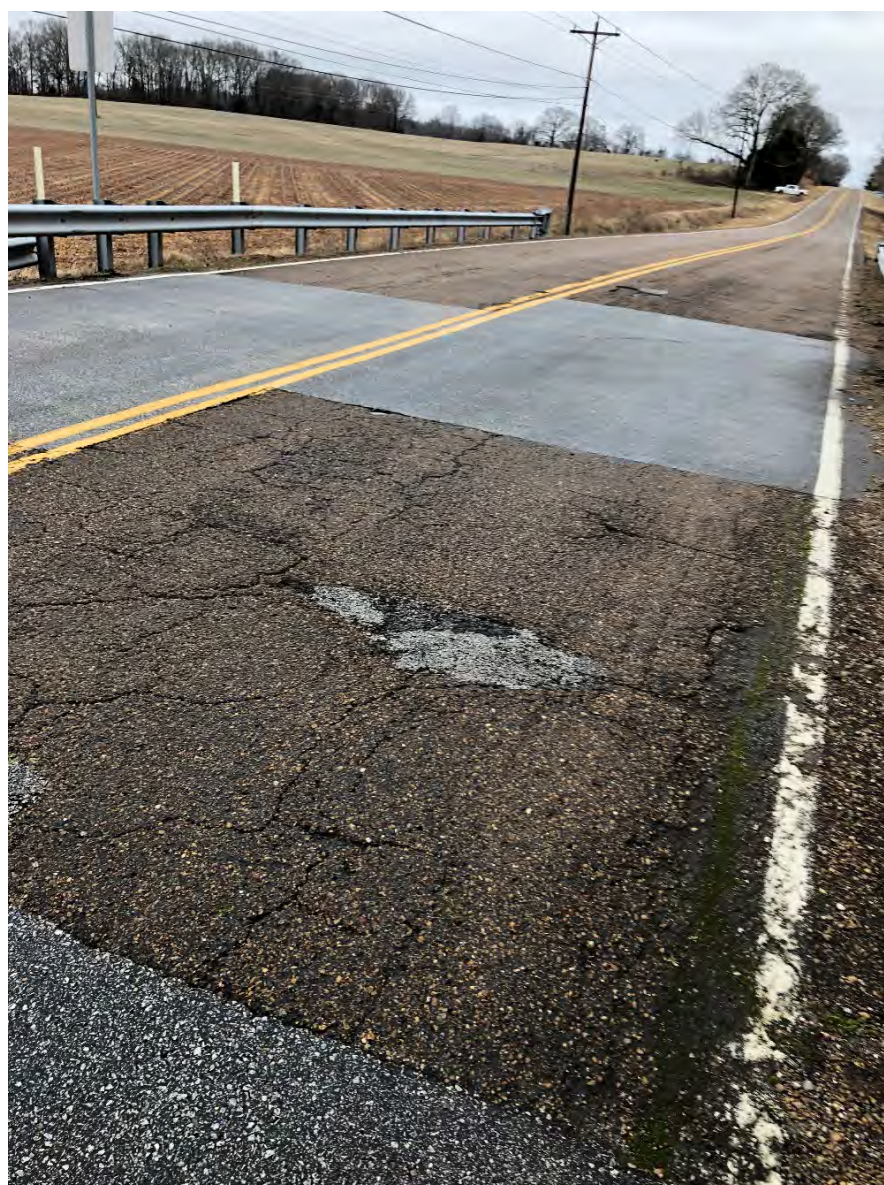
Spalling and Cracking along Surface
