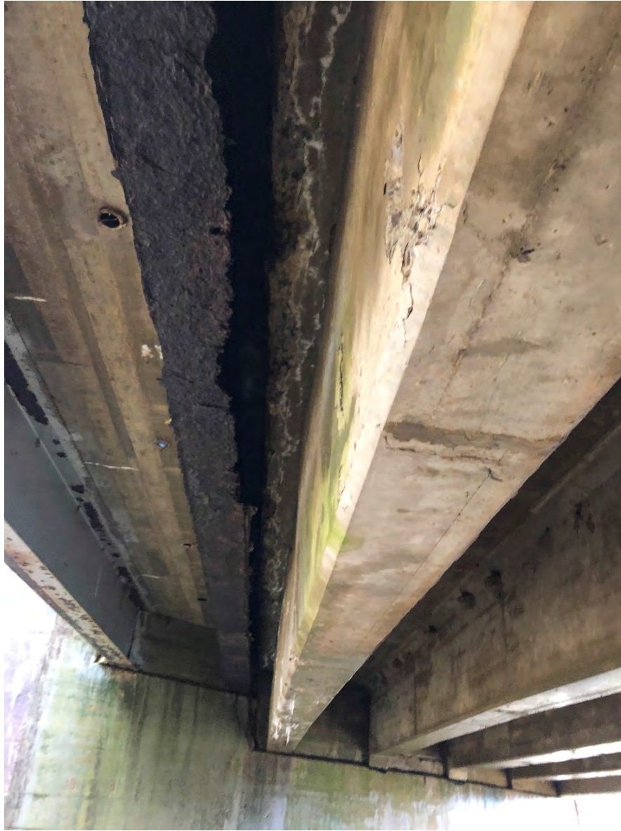
Extensive Corrosion of inner I-Beam at Inlet
