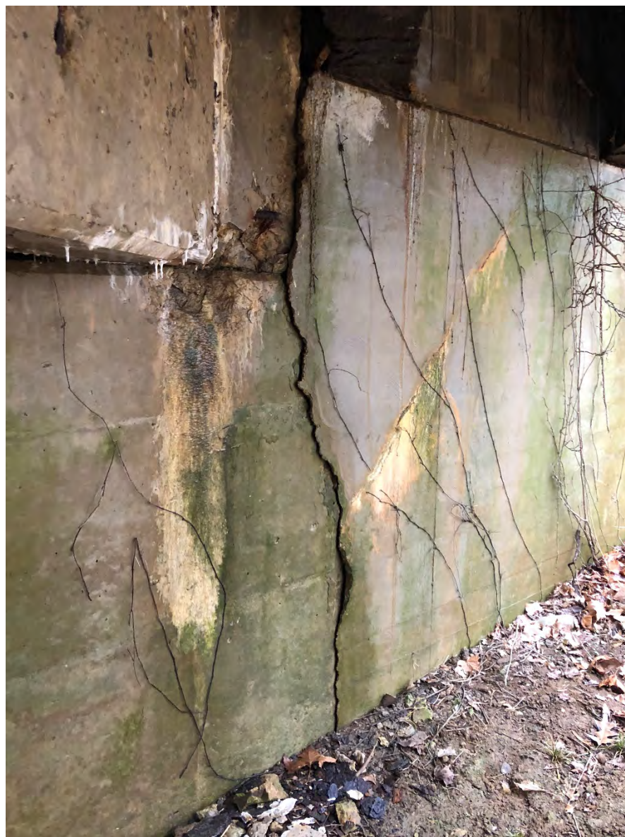
West Abutment Decay and Cracking
