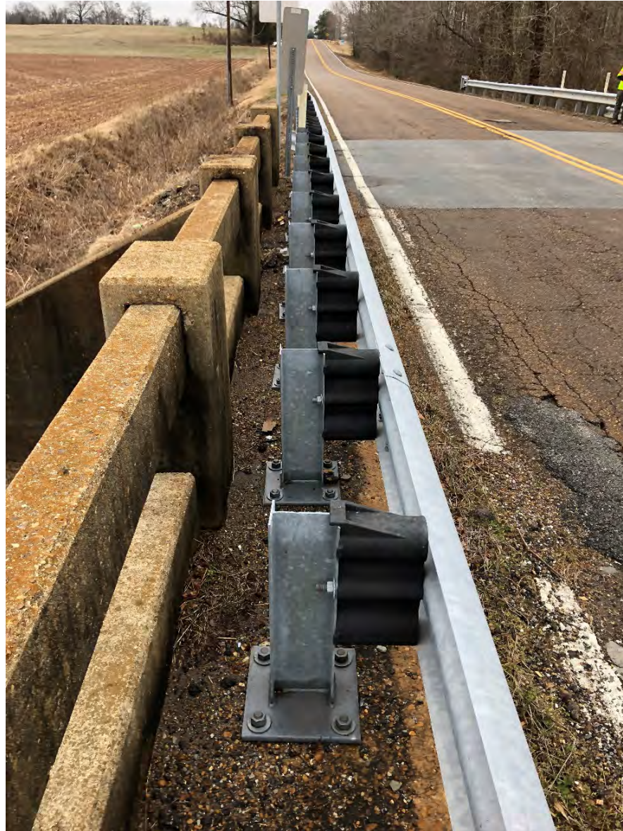
Poor conditions of Railing and Shoulder (Vegetation and Decay)
