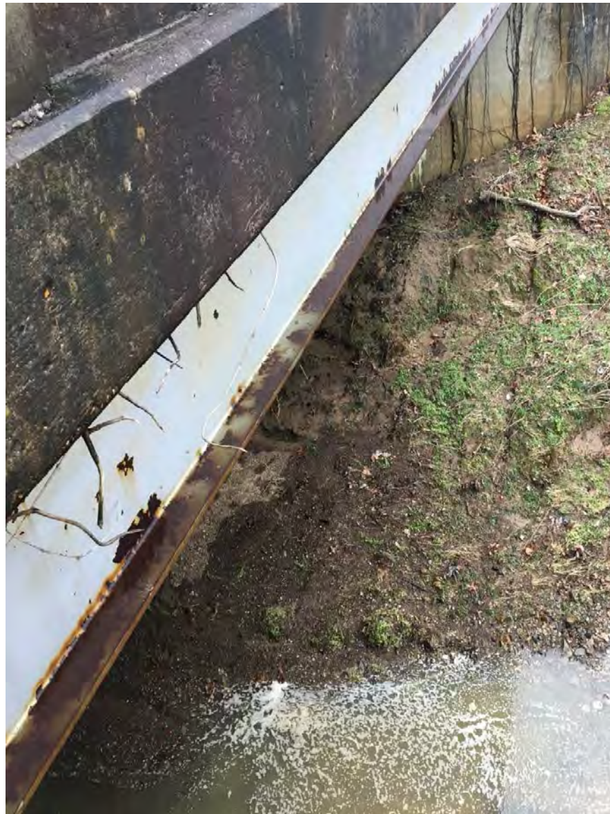
Severe Corrosion of Flange in Outer I-Beam at Outlet
