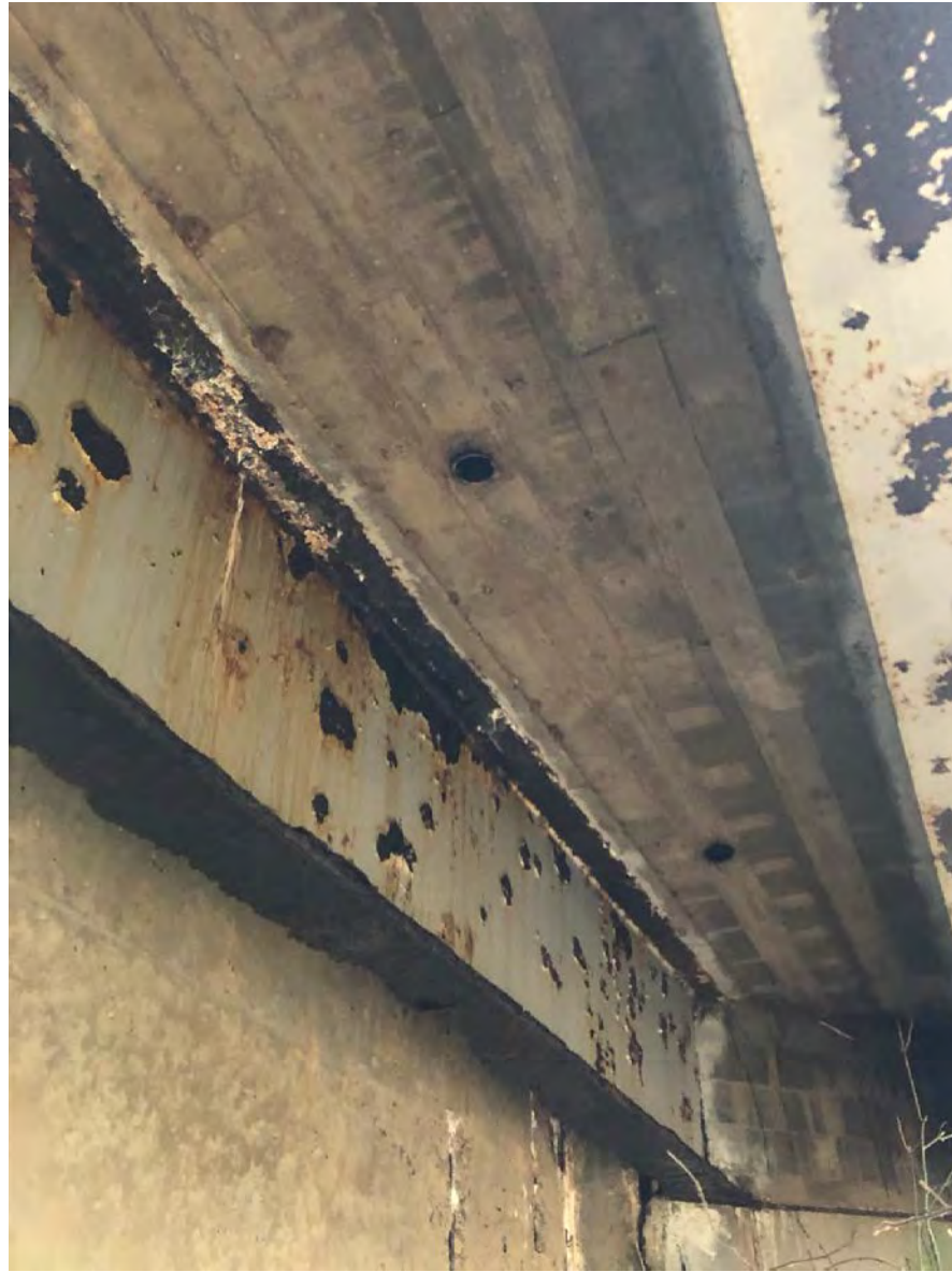
Extensive Corrosion on I-Beams at Inlet
